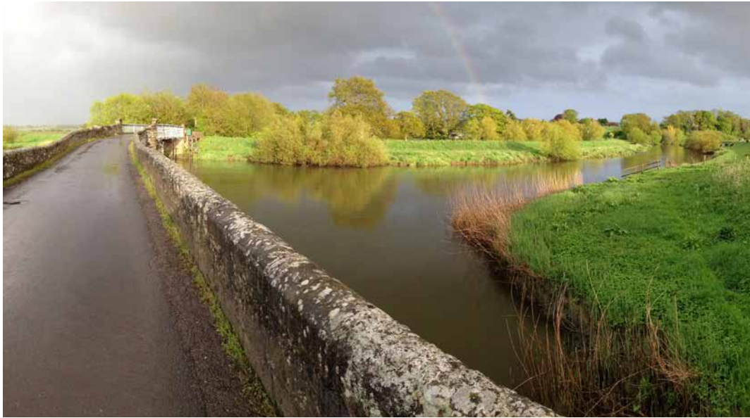
The National Park's roads and bridges form an integral part of its landscape. Greatham Bridge, Pulborough
