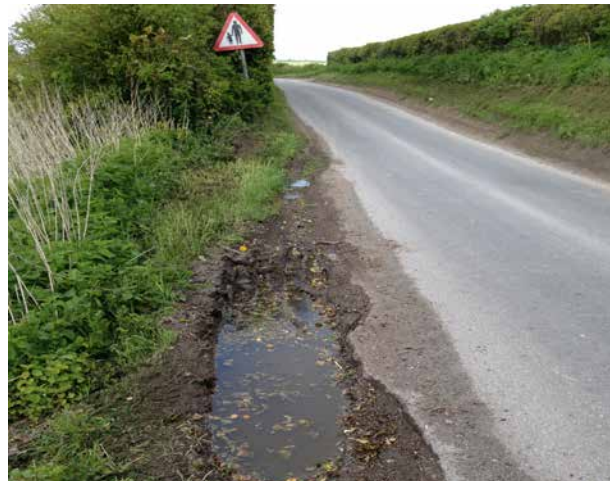
Damaged verge from poor edge detailing
